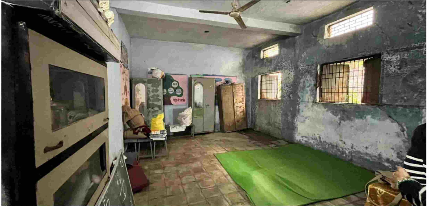
The government middle school in Hirapur, Sehore district, Madhya Pradesh. The school is located in a dilapidated building. It is in the same premises as the village panchayat office and a community centre ground. MEHUL MALPANI
